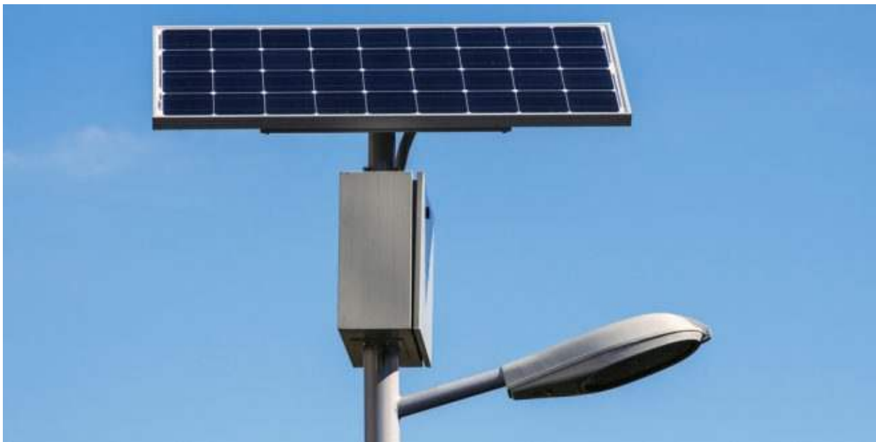
Figure 15 Solar powered street light with battery storage in box (Flood 2018)
